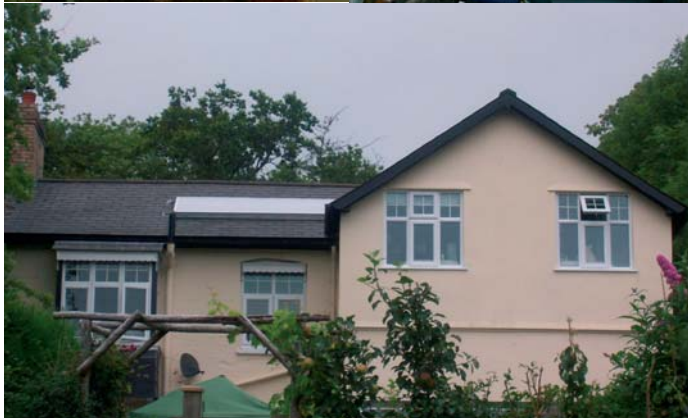
Airing cupboard with existing hot water storage tank and after with new thermal store for solar water heating installation on a house in Dulverton, Exmoor. (Top: Photograph courtesy of Ivan Gunn; Middle: Photograph courtesy of Maurice Shortman; Bottom: Photograph courtesy of Caroline Gunn)
