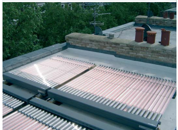
Evacuated-tube solar collector on the flat roof of Beaufort Gardens, a mid-Victorian terraced house in the Royal Borough of Kensington and Chelsea. (Top image: Photograph courtesy of Royal Borough of Kensington and Chelsea; Bottom image: Photograph courtesy of Claire Craig, English Heritage)
