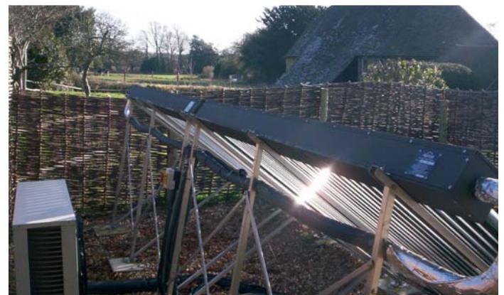
Ground-mounted solar collector at the Keeper's Cottage, Woolbeding, West Sussex, a timber-framed cottage dating back to the early 17th century, now owned by The National Trust. (Photographs courtesy of Robert Williams)
