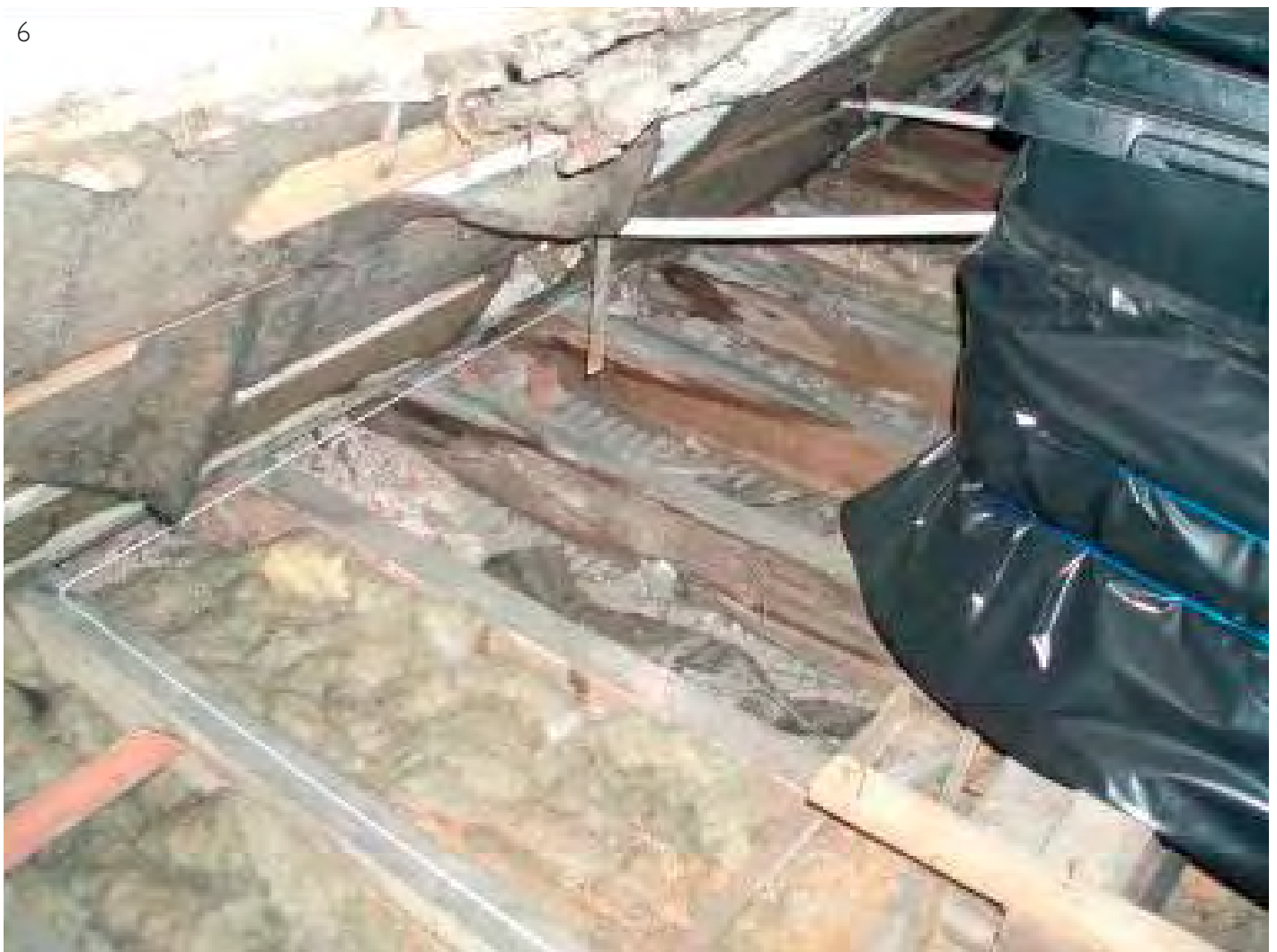
6 Missing insulation: make sure your insulation is complete. (Photograph courtesy of English Heritage)
